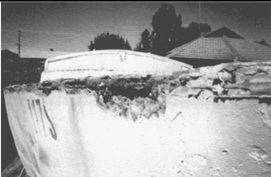
Extensive erosion along the deck joint
